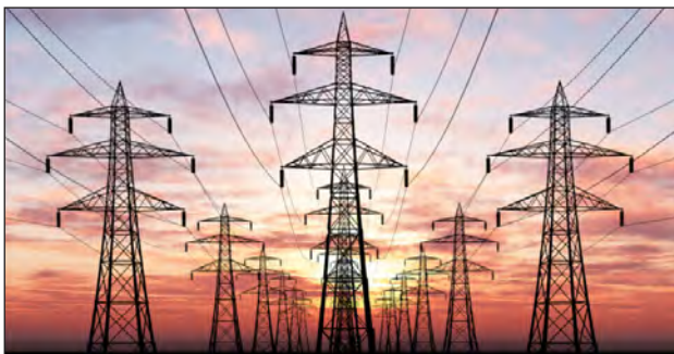
Electricity is transmitted along power lines to homes and buildings
